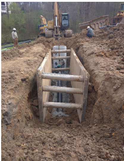
Rivergate Pump Station
