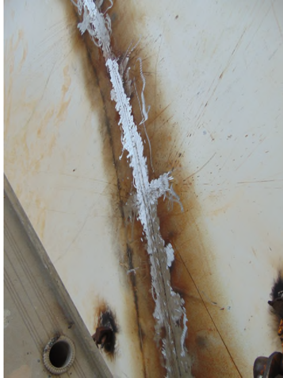
Photo #: 13 Description: Interior Wet: General view of S3 vertical joint.
