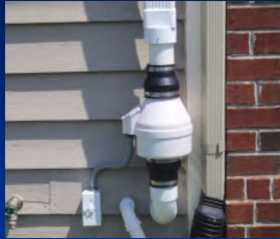
Fan with coupling from PVC to gutter downspout piping
