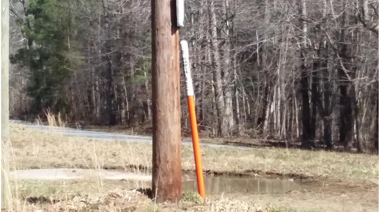
Fiber Optic Cable –North side of Route 6
