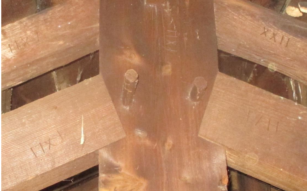
Figure 59. Detailed view of fabrication markings on roof trusses for use in assembly
