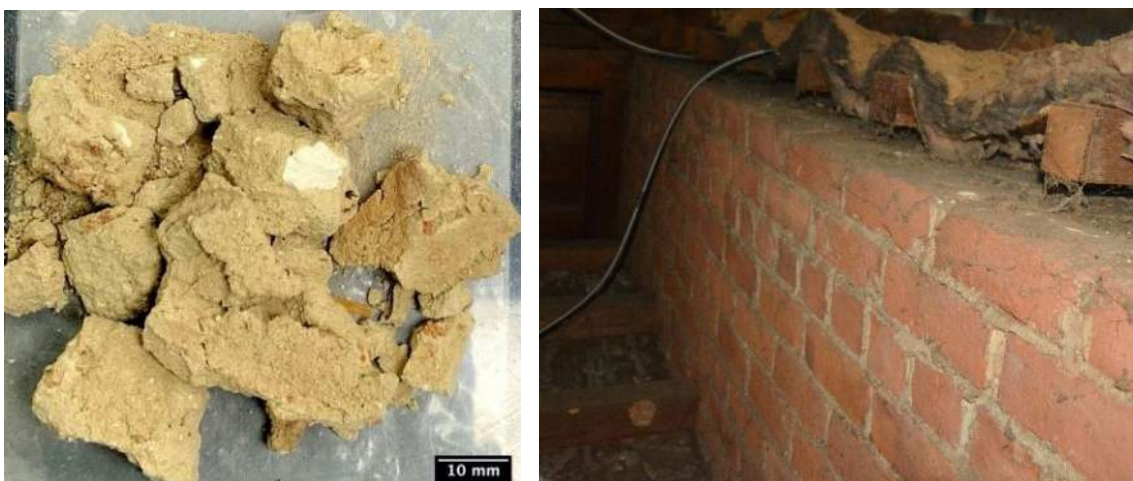
Figure B9. Mortar sample FM-01 and location from south elevation brick wall exposed in attic.
