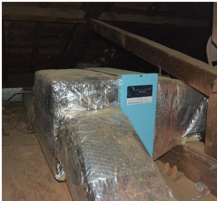
Figure 55. View of mechanical unit in attic
